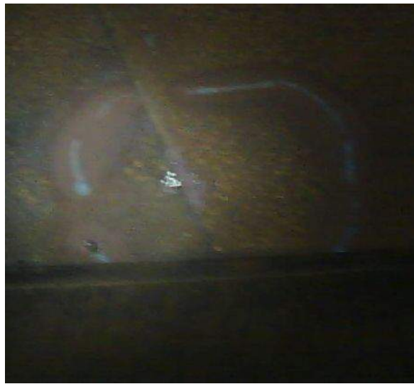
Photo #1 - Underside of Tank Roof Where Burn-Through Occurred
