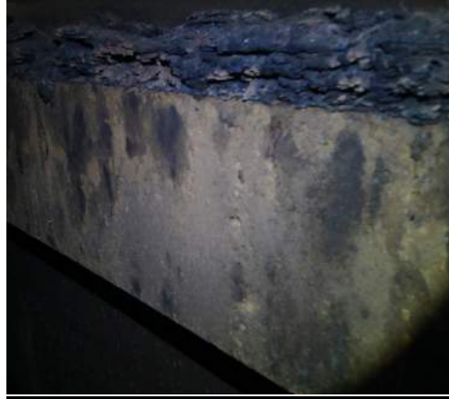
Photo #2 - Corrosion Material Build-Up on Upper Reinforcement Ring
